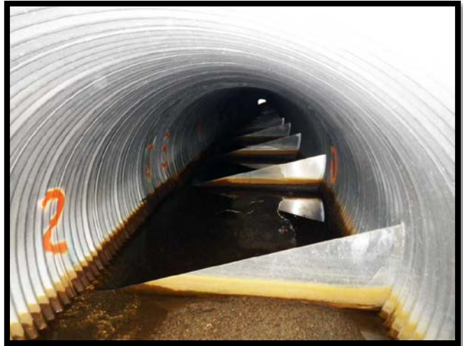
Figure 1. Shows a culvert with baffles installed. These baffles mimic waters natural flow by reducing flow velocity allowing fish to swim upstream.
