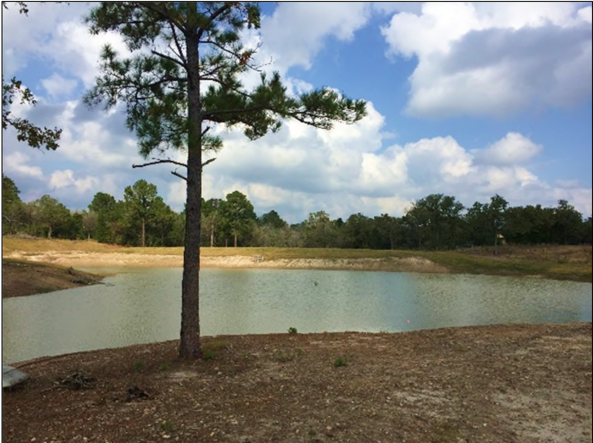
Photo 3: One of the four grade stabilization structures completed through the project. This structure was implemented by Donald Sly in Fayette County.
