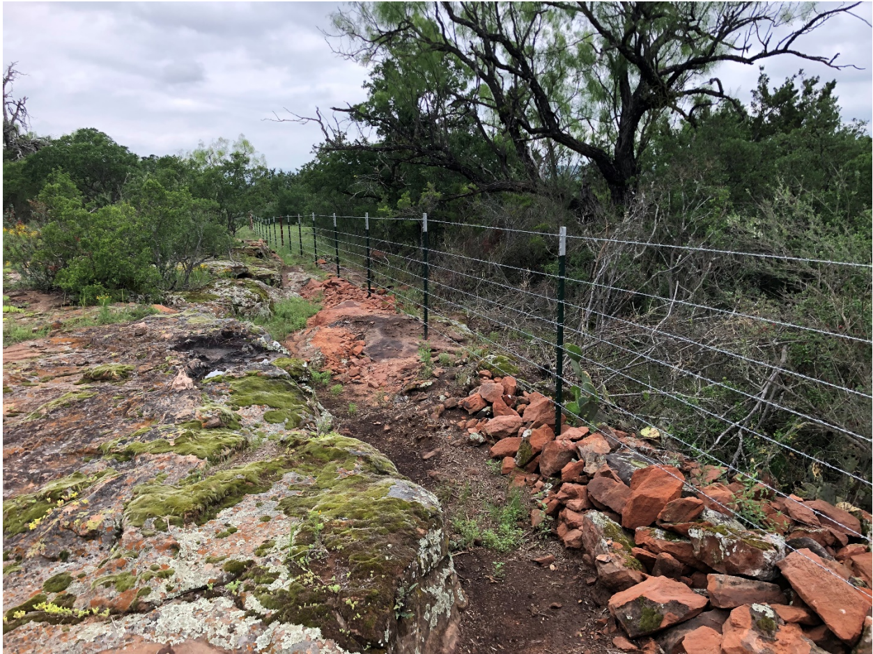
Photo 1: Features a 3,648 ft. cross fence installed in Llano County. The fence allowed the producer to rotationally graze their livestock and was in the “Steep, Rocky” payment category.
