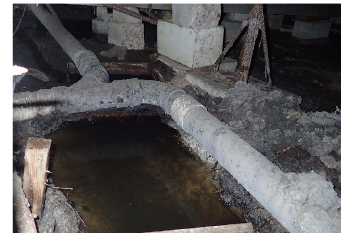
FIGURE 2.1 Pooling wastewater above septic tank in the Tres Palacios Creek watershed (Photo by Ryan Gerlich, Texas A&M Agrilife Extension Service)
