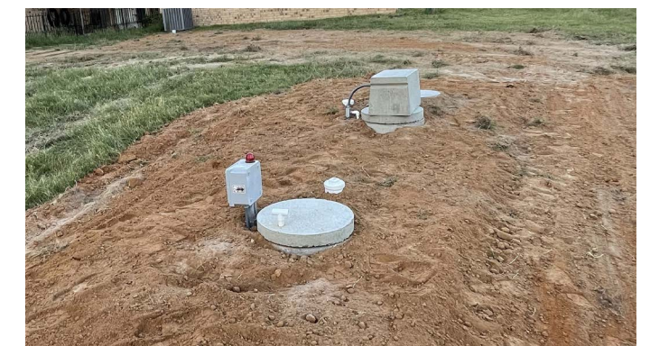
FIGURE 2.2 New septic system installed with proper sloping to prevent standing water from damaging pump (Photo by Eddie Sifuentes, CL Septic)
